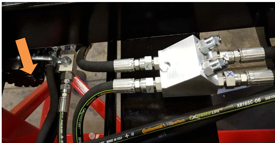
Figure 11: Manual bypass valve
